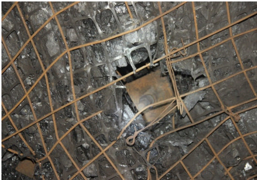
顶部锚杆被勒入顶板
